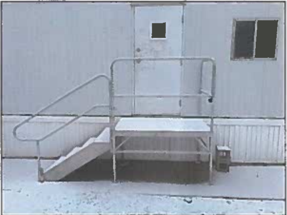
Door 1 with Existing Steps
